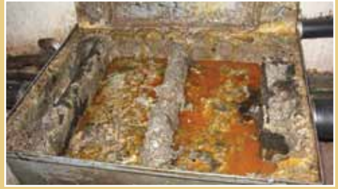
GRD too full of FOG and not maintained properly.
