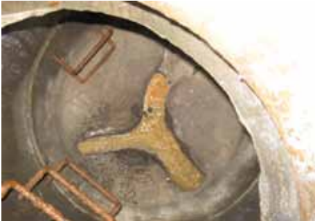
Grease clog in sewer.
