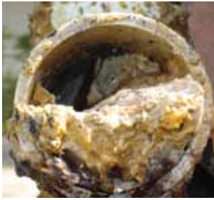
Grease clog inside a pipe.
