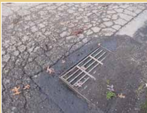
Standing water due to clogged drains can damage pavement.
